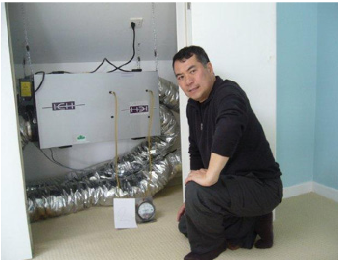
Super E® Member Arthur Lo preparing a ventilation balancing test with a newly-installed ERV.
