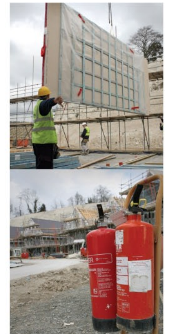
IFC has put the scheme forward for the Fire Safety Engineering award sponsored by Wagner Sprinklers.
